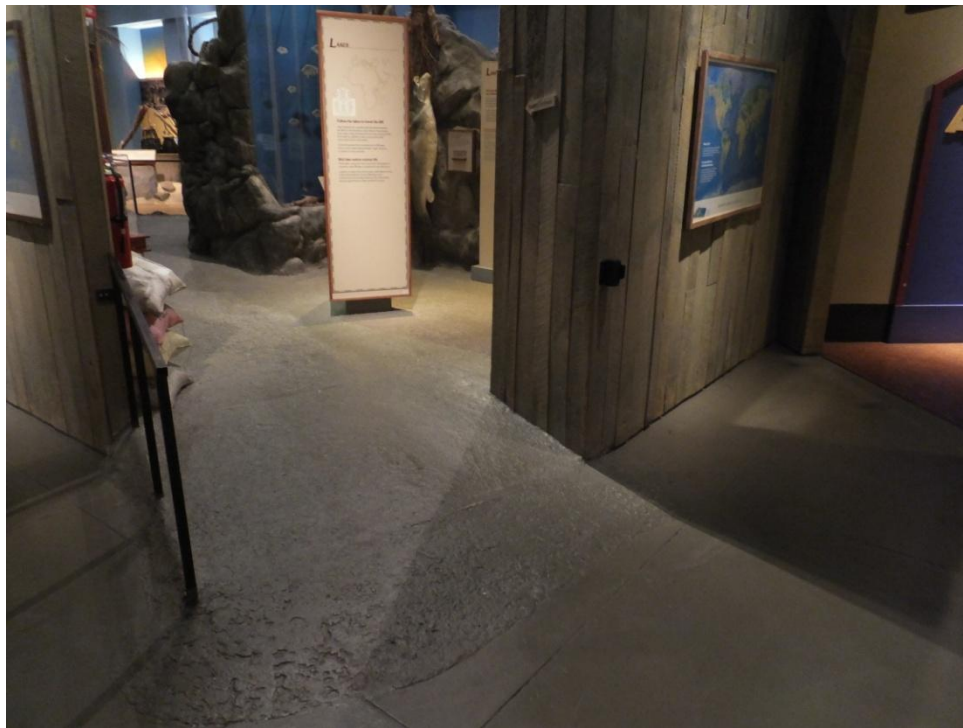
Figure 52 -- Ramp at Africa Exhibit (Lakes Display) has steep 11.0% Slope
